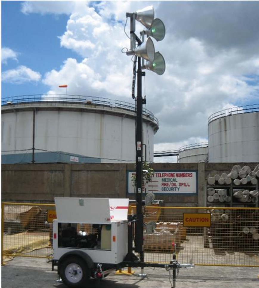
Mobile Lighting System with Diesel-driven Generator
